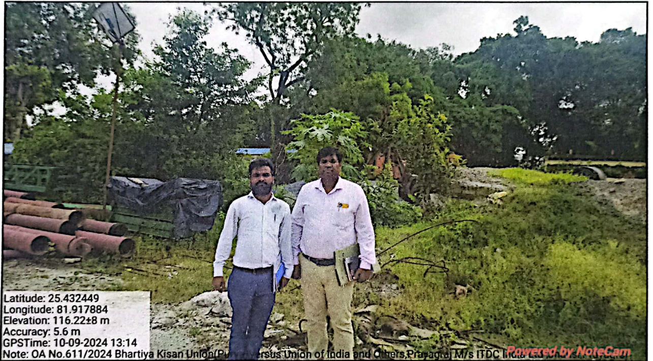
Photographs showing dismantled concrete batching plant of M/s ITD Cementation India Pvt. Ltd. , Jhunsi, Prayagraj on dt. 10.09.2024.
