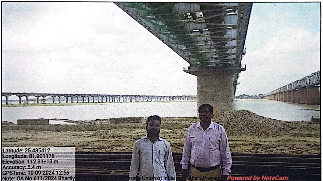
Photographs showing newly constructed Rail bridge over River Ganga near pier no. 01 towards Jhunsi, Prayajraj on dt. 10.09.2024.
